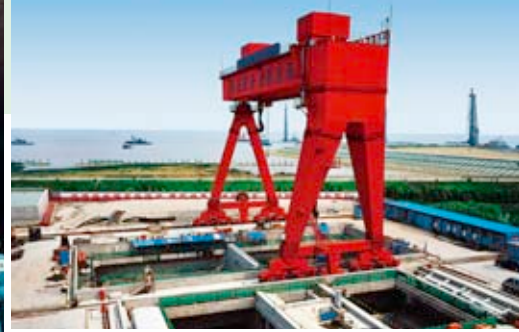
Launch shaft of the S-317, S-318 on the banks of the Yangtze river.
